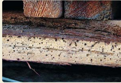
Insect damage on wooden pallets
